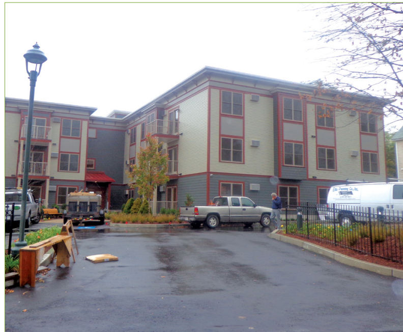
Winter Gardens Apartments, Quincy
